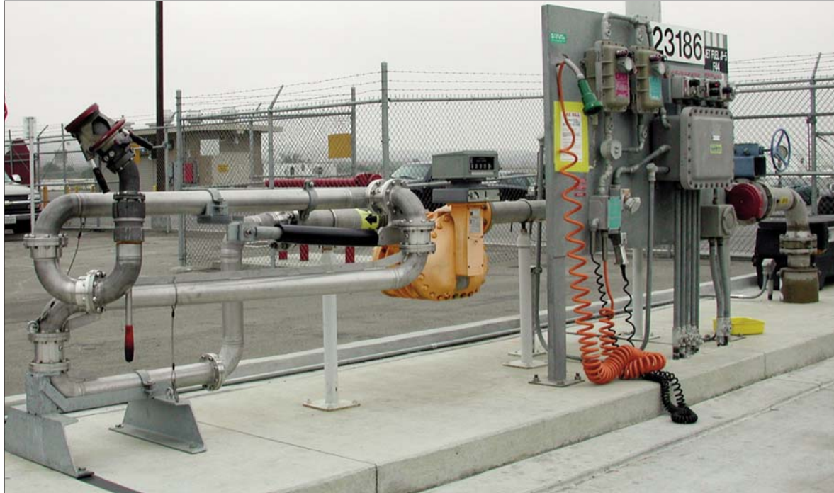
Refueling of tank trucks with bottom loading connection
